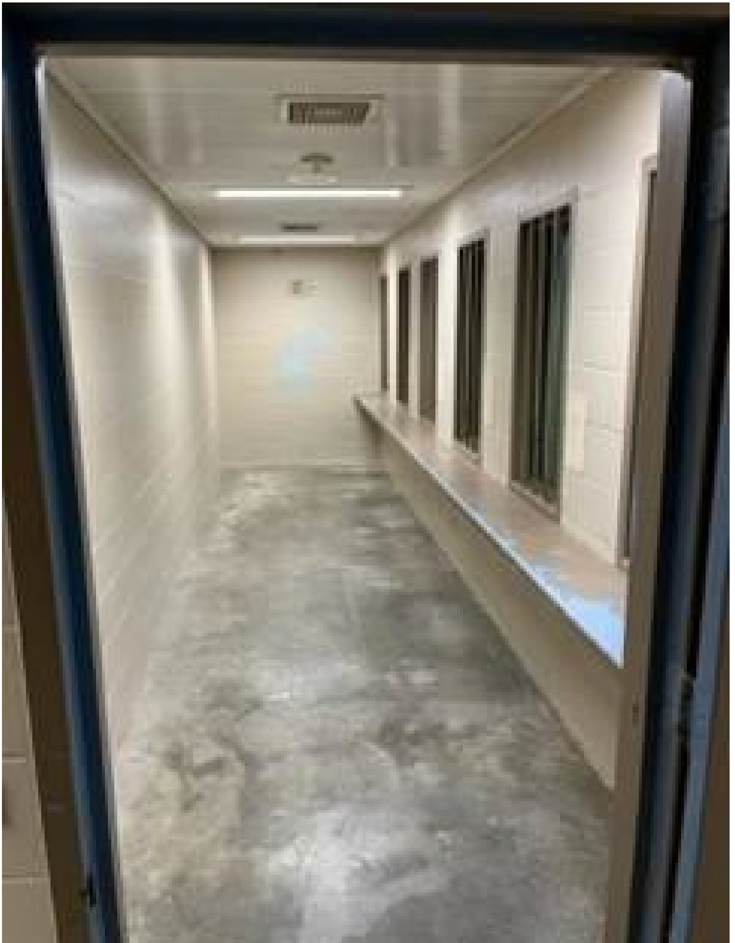
"MEDICAL OBSERVATION" CELL WITH NO TOILET OR WATER
