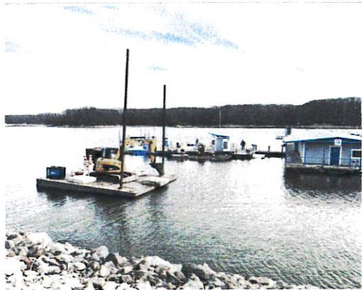
Lithia Springs Marina Gas Dock Anchoring
