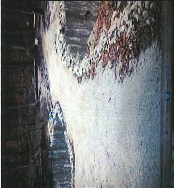
This pic was taken today at lake level 612.6. The newest projection is to crest at 619. The trail is closed. The culvert will go under at 614.
